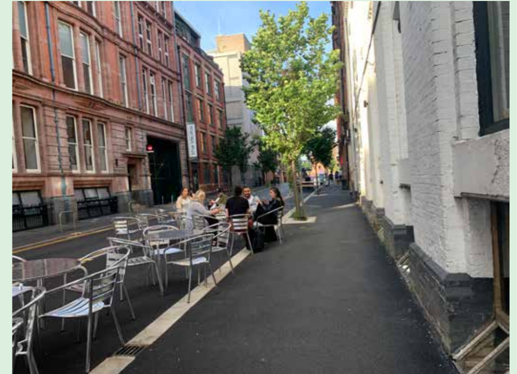
Footway widening in Tarrif Street, Manchester to allocate additional al-fresco dining areas
